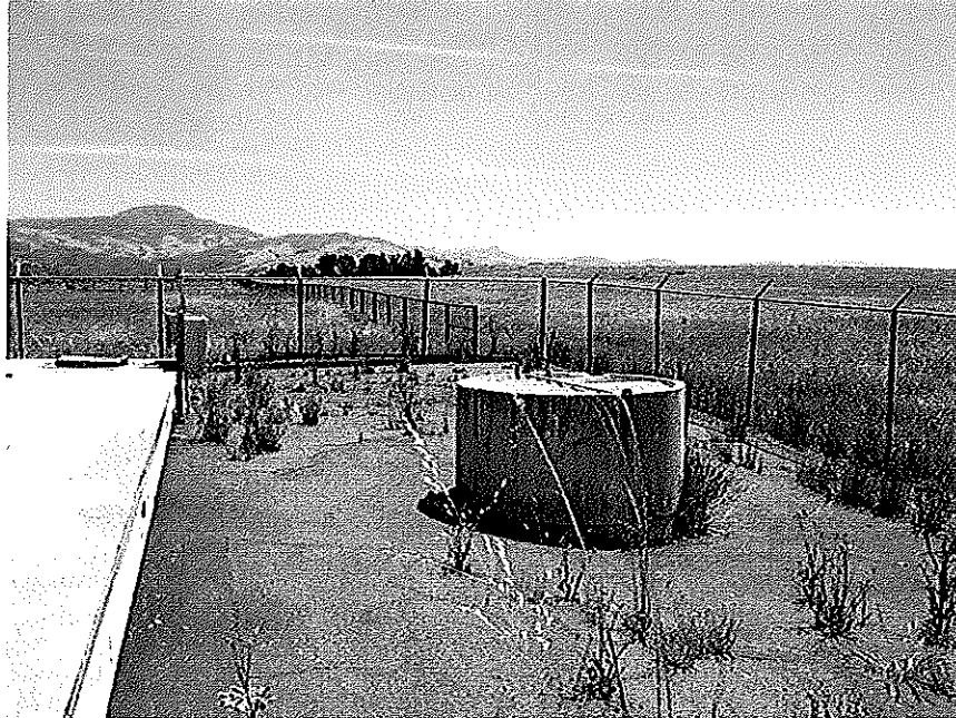
Photograph #19: View from Facility, Looking East – Altitude Valve in Foreground
