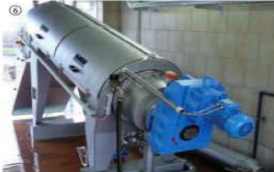
Sludge dewatering for surplus sludge treatment, > 18 % DS
