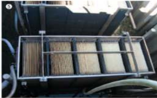
HUBER BioMem® filtration unit installed in a container as a decentralised solution
