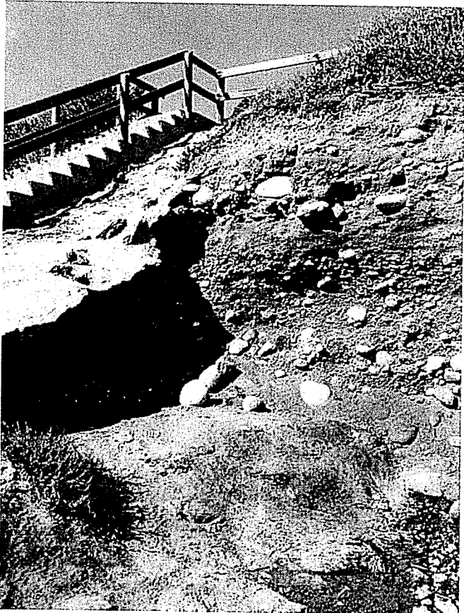
South side of staircase showing another view of undermining/erosion.
