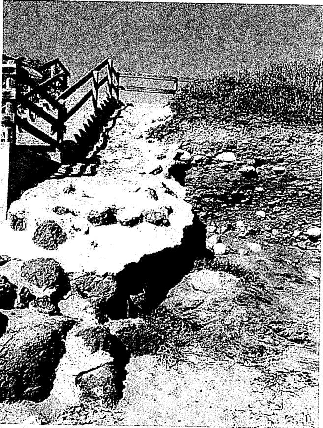
South side of staircase showing undermining and erosion.
