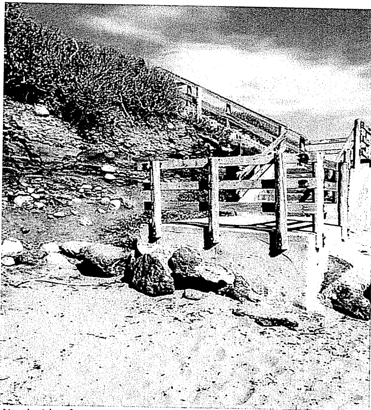
North side of staircase showing concrete landing and bluff erosion.
